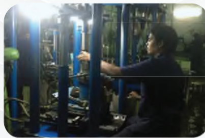
DEEP WELL MOTOR SETTING
